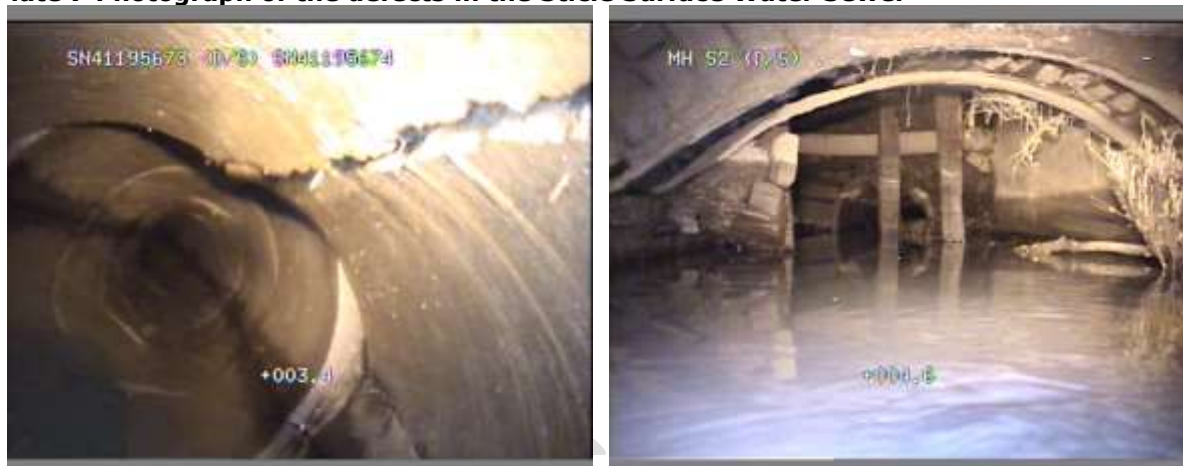
Plate 7 Photograph of the defects in the Sticle Surface Water Sewer
