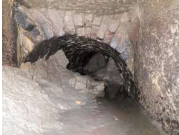
Plate 6: A partially blocked surface water sewer off Old Llangunnor Road, Pensarn.
