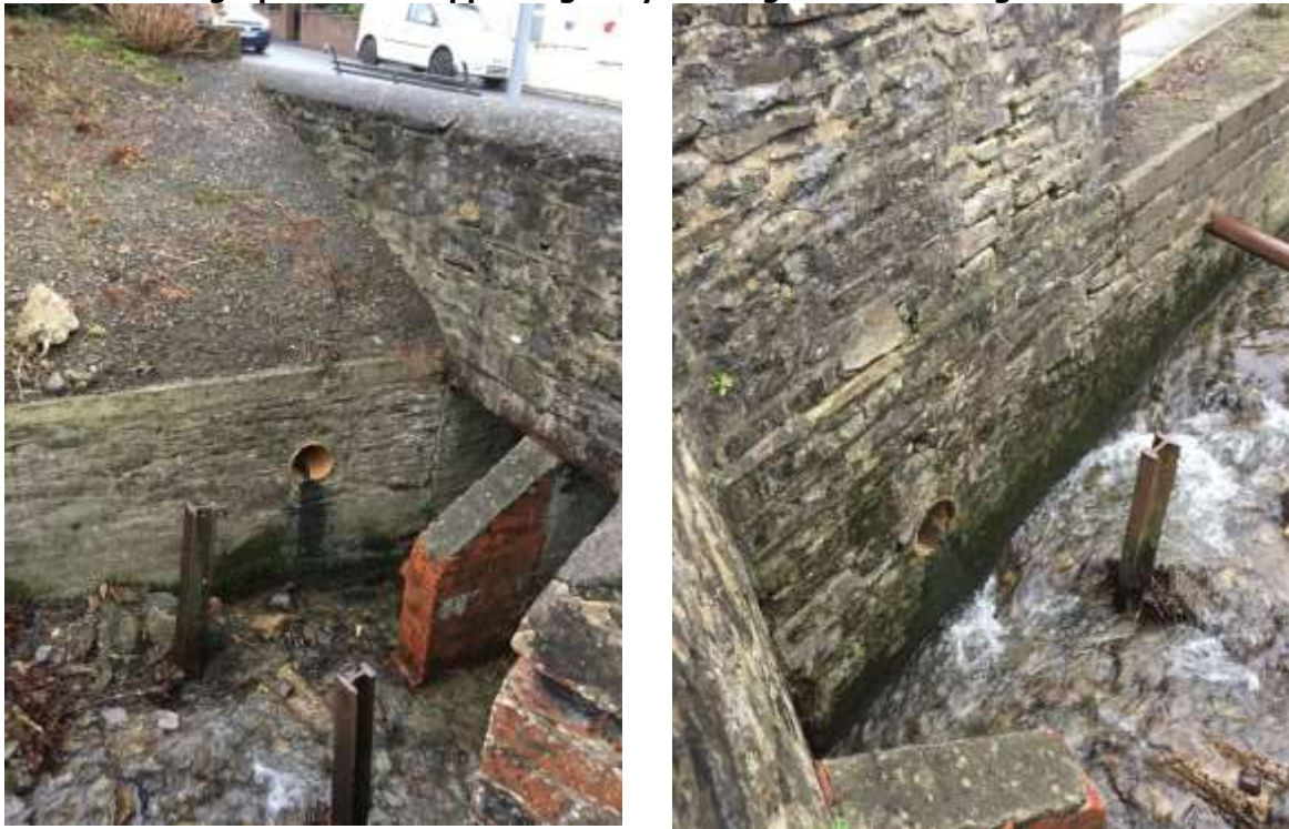
Plate 10 Photographs of un-flapped highway drainage outfalls along the Nant Einon.
